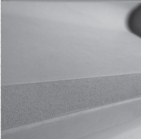
GIAN T02 concrete stair nose
